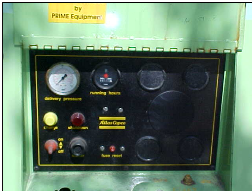
Figure 4 – Air Compressor Control Panel
