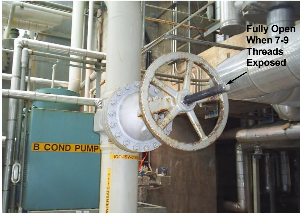
Figure 1 - Condensate System Discharge Valve
